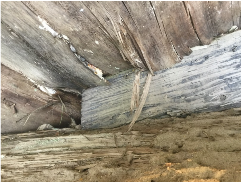
Stringer 3 Right Abutment Crushing of Sap Wood
