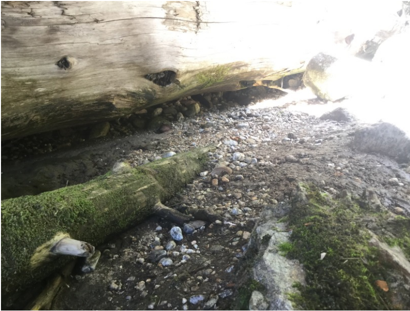
Scour Under Right Abutment Log
