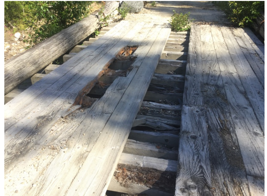
Rotten Deck Planks and Ties
