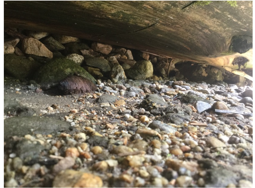
Scour under Right Abutment
